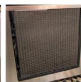
3=Due for cleaning
