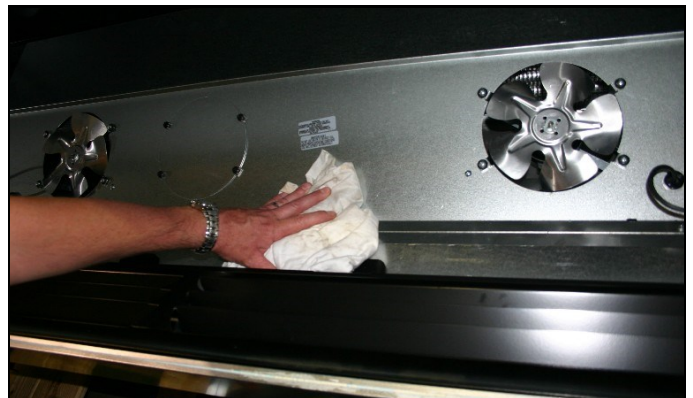
Image #2 Clean under air return grille and fan shroud area with moist cloth. Remove drain cleaning access door and clean drain.
